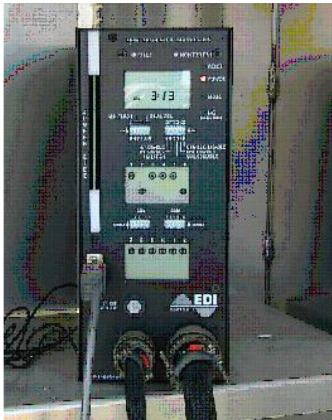
Figure 12.5 – Typical conflict monitor
